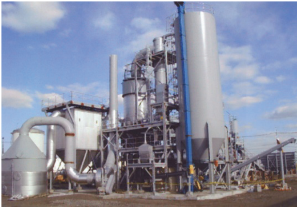
Rotary kiln air treatment system
