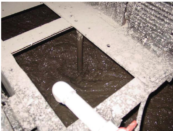
HREG chemical mixing tank
