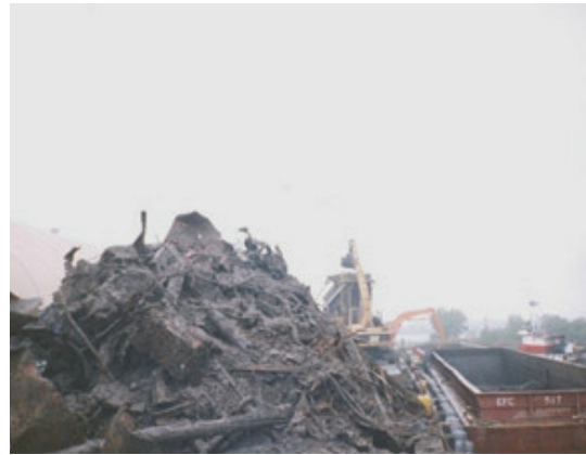
Debris pile from harbor job
