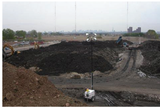
Interim PDM storage facility
