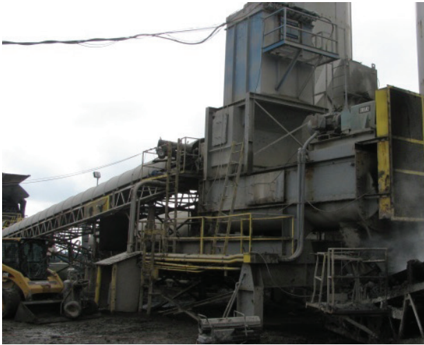
Conveyor feed single pugmill system
