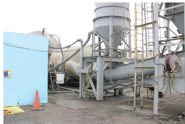
Pneumatic pozzolan metering system
