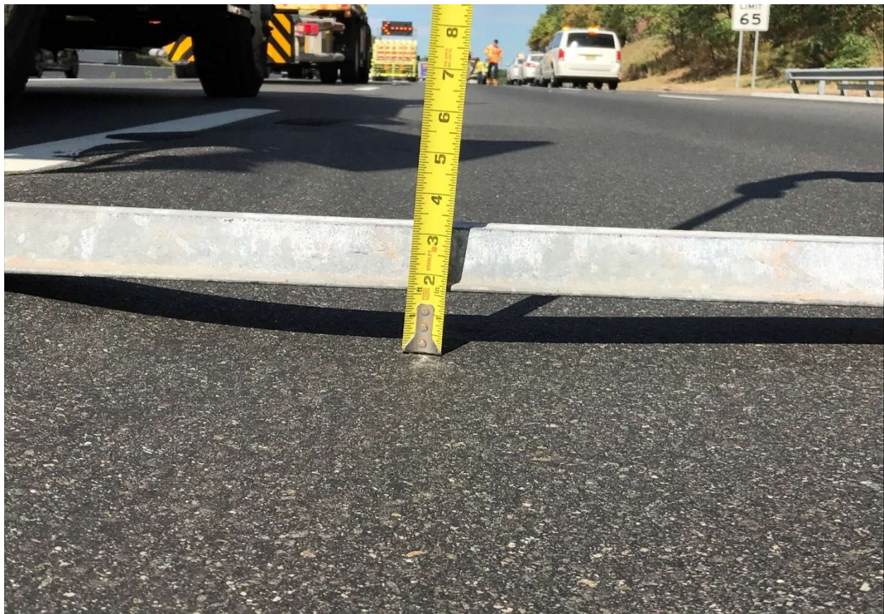
Figure 7a. – Asphalt Rutting in the Wheel Path that Requires Repair
