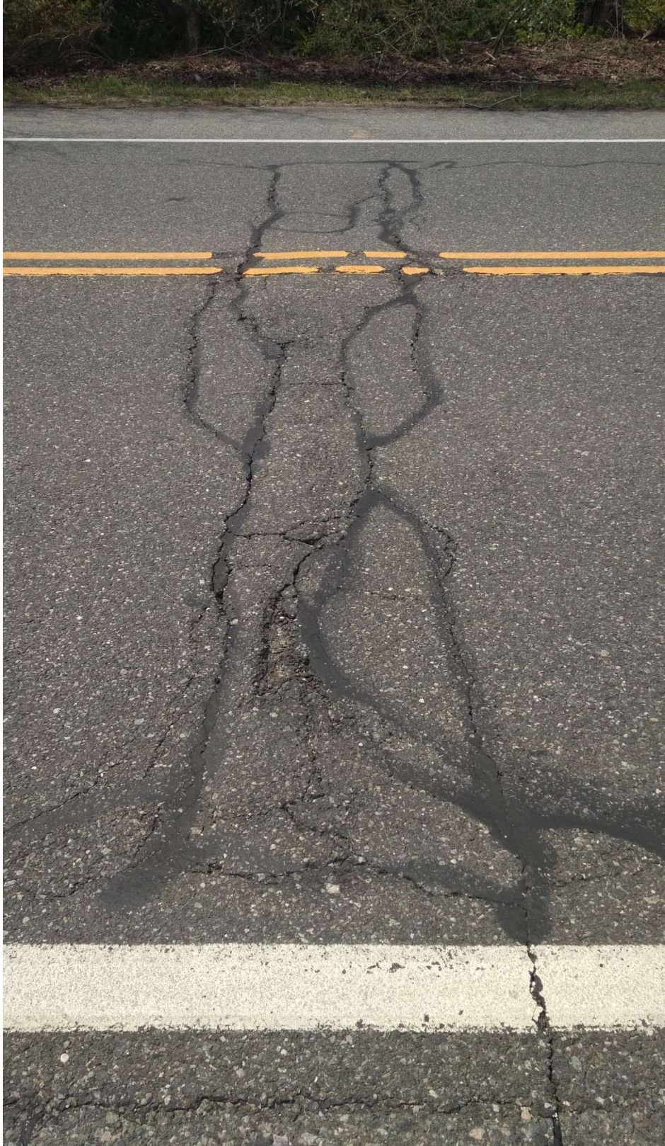
Figure 6 – High Severity Reflective Cracking of Asphalt over a Concrete Pavement Joint (Composite Pavement) Area Requiring Repair
