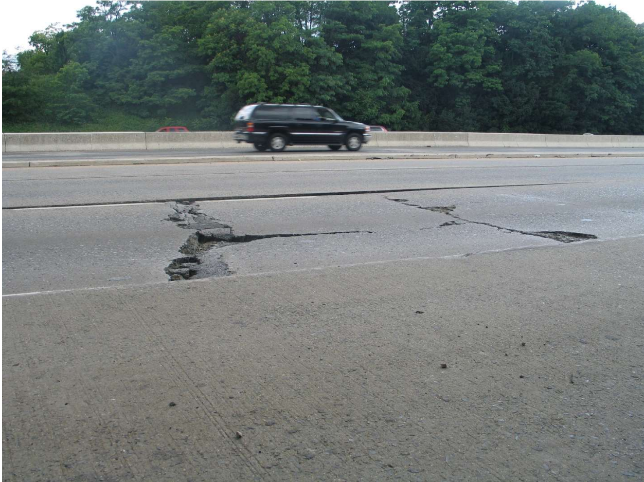
Figure 9 – High Severity Concrete Distress (High Severity Cracking, Spalling, Potholes and Faulting) Requiring Full Depth Slab Repair
