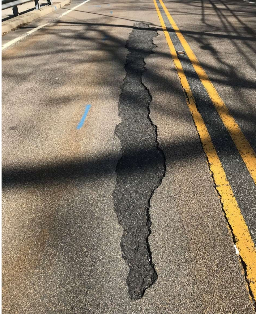
Figure 4 – Failure of HFST and Asphalt Substrate
