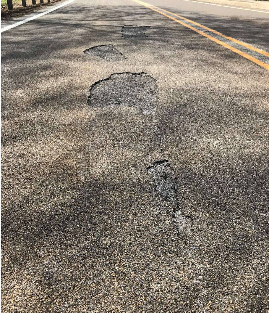
Figure 5 – Failure of HFST and Asphalt Substrate
