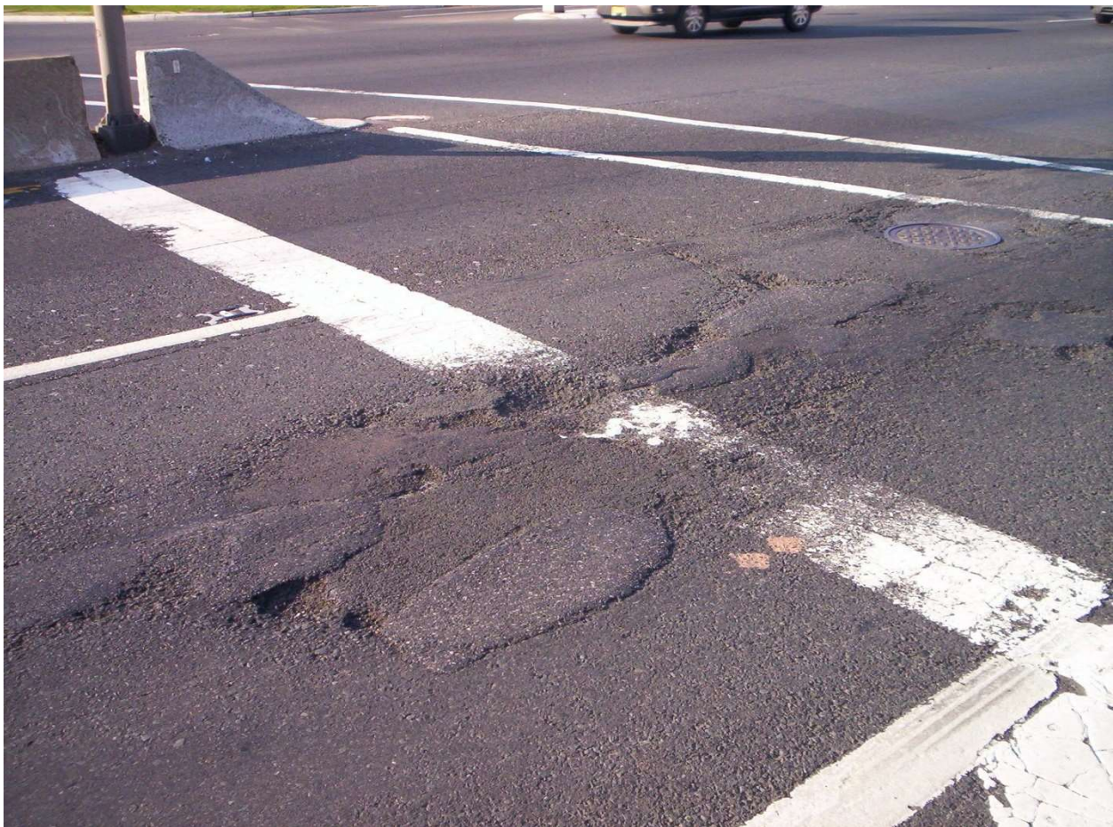
Figure 8 – Asphalt Potholes, Unsound Patching and Raveling Requiring HMA Pavement Repair or Milling and Resurfacing
