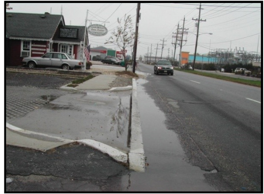
Ship Bottom drainage issues
