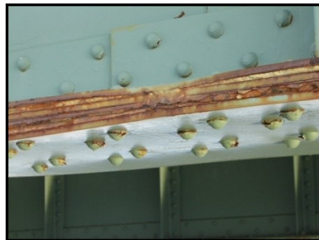
Pack rust delaminating bottom flange
