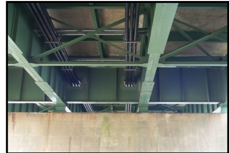
Utilities on the Bay Bridge
