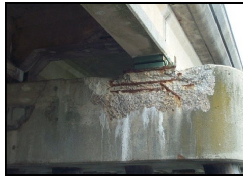
Pier cap failure on trestle bridge
