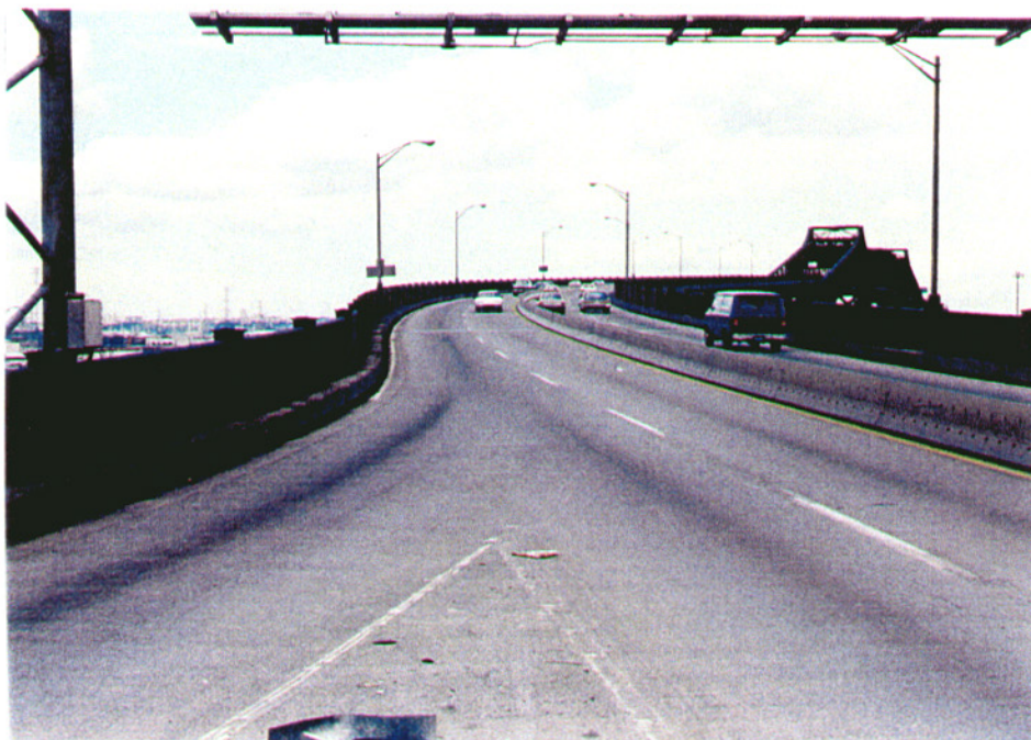
b) Typical roadway and railing configuration on high-level viaduct of Pulaski Skyway in Newark.
